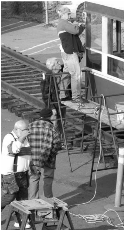
The first of the windows goes up to help temporarily protect the Birney Car - Photo by Robert Baxter
