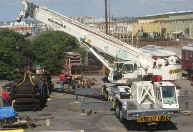
A crane moves snap track around in the yard prior to moving the MOW vehicles onto Track 2. Photo by Robert Baxter
